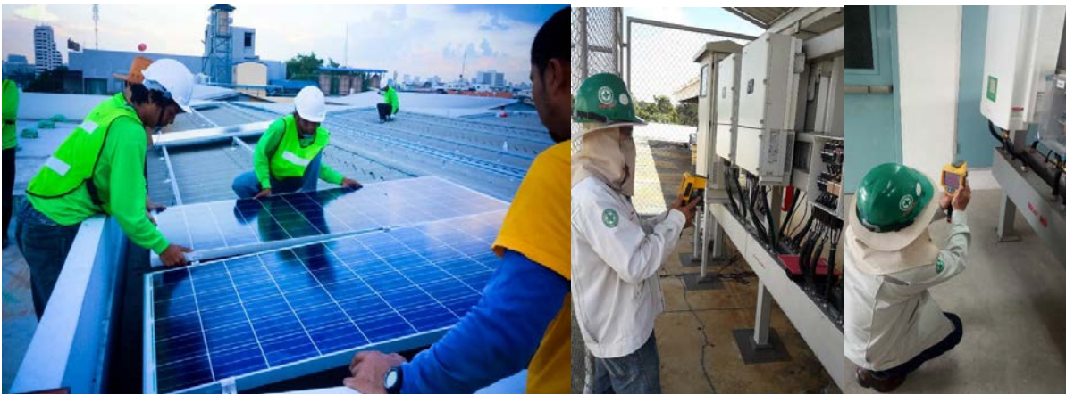
Operation & Maintenance Service
