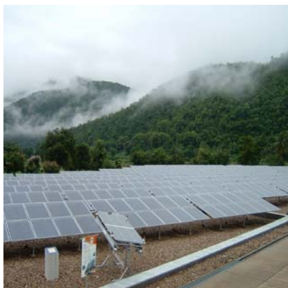
500 kWp, Mae Hong Son Province.
