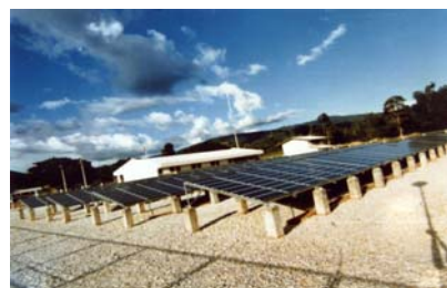
40 kWp, Tak Province.
