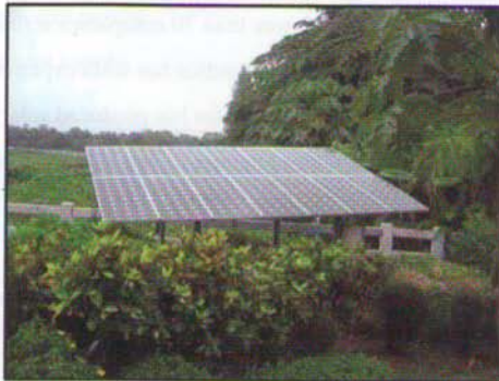
Solartron solar panels
